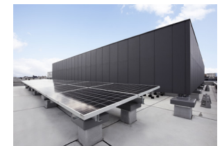
Solar panels installed on the rooftop of Oakwood Hotel Oike Kyoto
